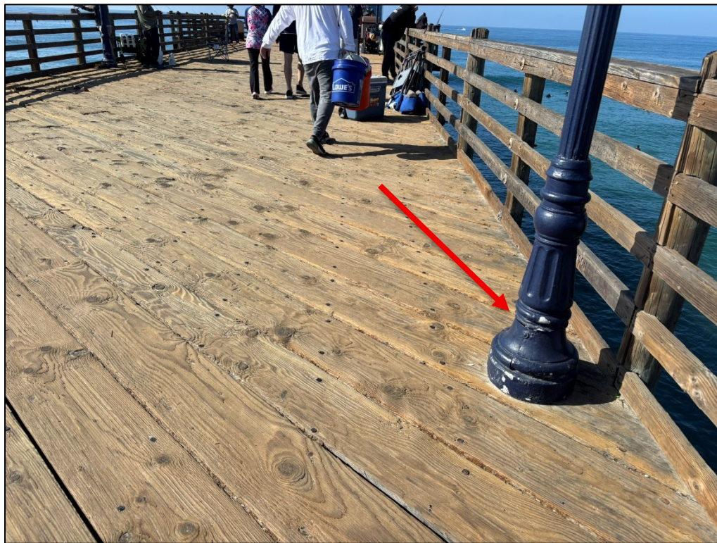
Photo 1. Light Pole, typical of four locations (Bents 18.5, 20.5, 22.5, 24.5) to be removed and reinstalled by City and Contractor, see Specifications.
