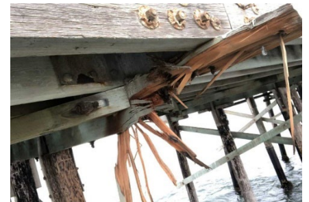
Photo 4: Balboa Pier Damage Assessment
