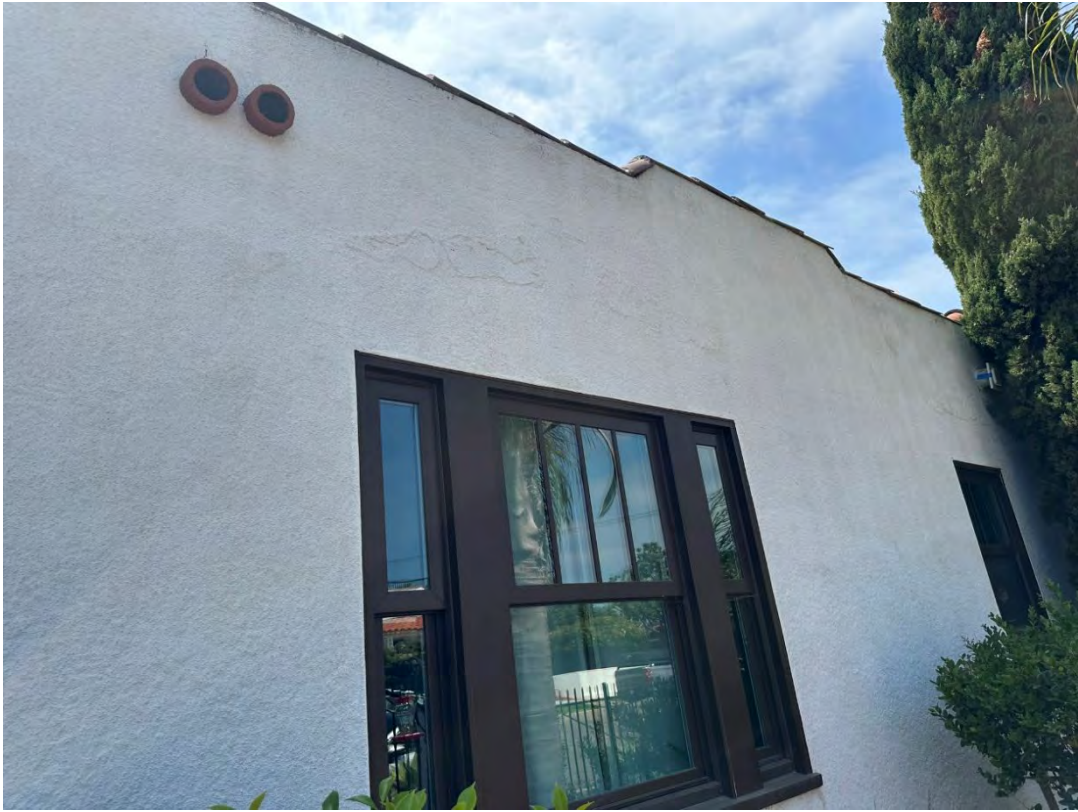
Above: Close up of original embellishments still visible on east elevation
